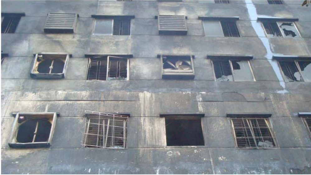
Caption: Tazreen Fashions Limited Building after the fire (Photo: Odhikar)
