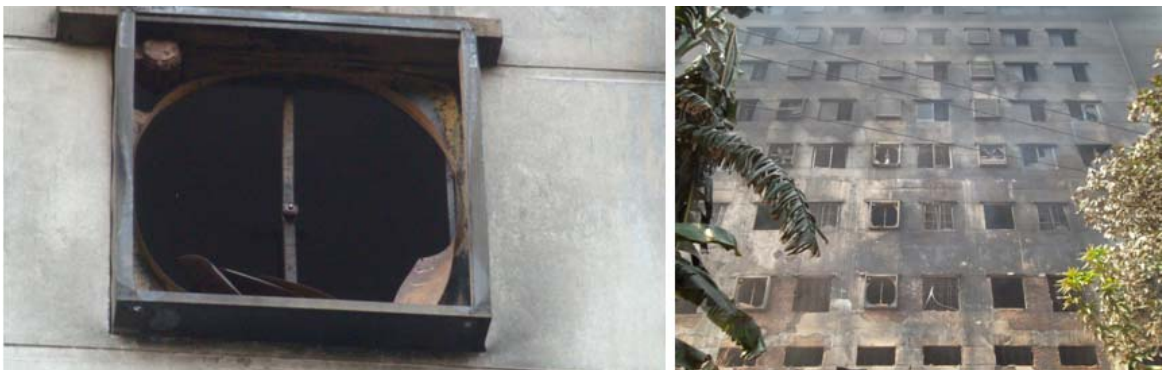
Caption: Broken exhaust fan, from where Nargis and other workers jumped to ground (Photo: Odhikar)
